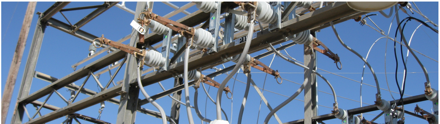
Substation field imagery from the Apex services website [P6]
